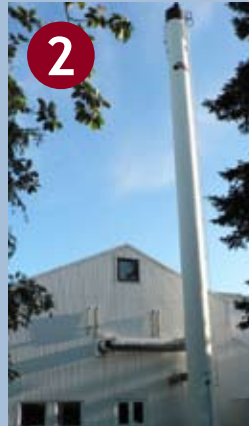
2 FRØSTRUP Heating plant (waste wood)
